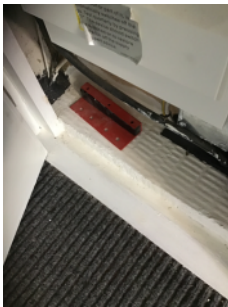
Fire stopping within electrical meter cupboards.
