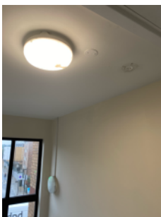
Maintained EL is provided in the staircase
