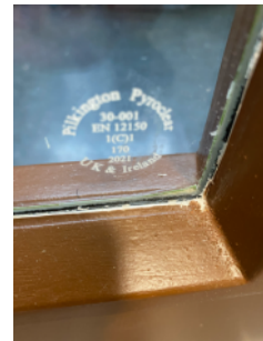
Acid etching on FR Glazing installed in lobby doors
