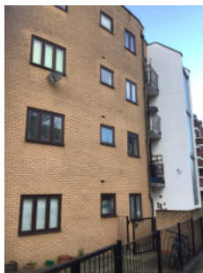
Brick/mortar external walls, with rendered section around the staircase External wall details
