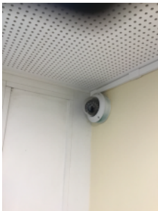
CCTV is provided in the entrance lobby.
