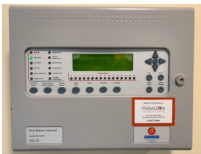
Panel for smoke detection for AOV actuation
