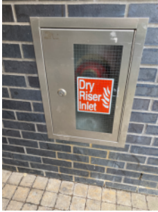
Dry riser inlet located outside main entrance door
