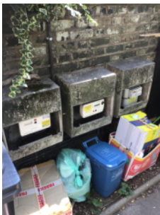
Gas meters are located externally.
