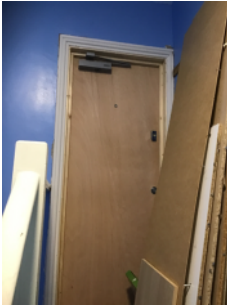
Example of combustibles on the common escape route.
