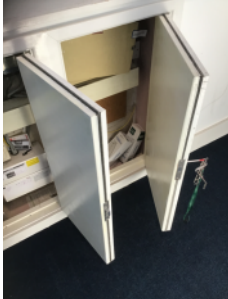
FD30S Doors fitted to the electrical cupboard
