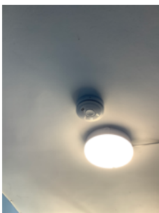
Part 6 fire alarm in common areas.
