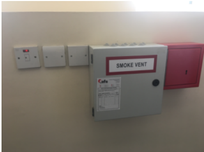
Smoke vent control panel.
