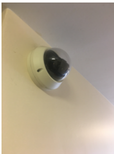
CCTV is provided internally and externally
