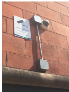
CCTV is provided internally and externally
