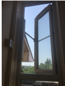
Window AOV on the 3rd floor defective in open position
