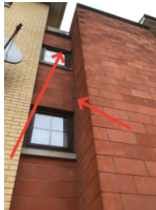
Indicating where it appears this section is a vertical hung tile system
