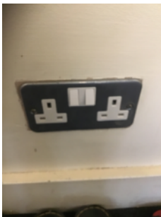
Electrical sockets within the staircase
