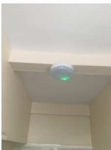
Maintained EL provided in the entrance hallway
