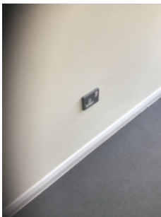
Electrical sockets provided in common areas
