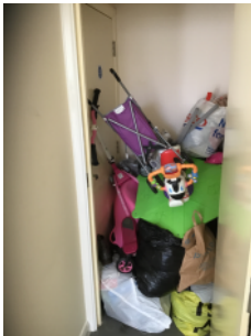
High volume of Combustibles in riser cupboard
