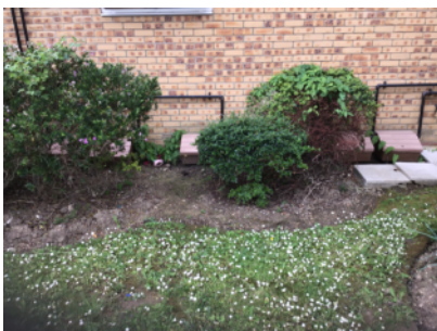
Gas meters located externally
