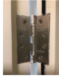
CE1121 marked fire rated door hinges fitted on electrical cupboard door
