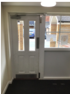
No exit signage over main entrance door.
