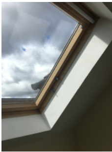
Window AOV appears defective
