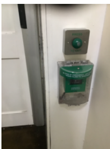
Door release and emergency door release.
