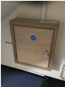
New FR enclosure
