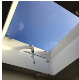
AOV in staircase
