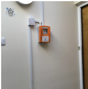
Smoke vent control panel
