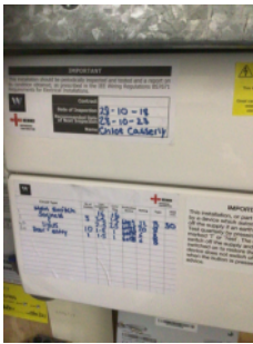
Evidence of electrical installation testing.
