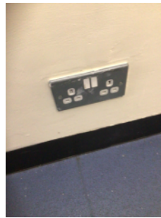
Electrical sockets are provided in the common areas
