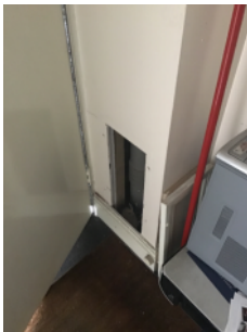
Opening in pipework enclosure in entrance hallway.
