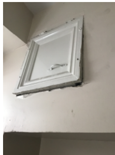
Opening in pipework enclosure in entrance hallway.
