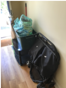
Combustible items present on the common escape route.
