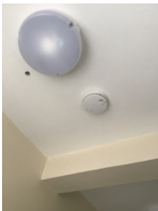
BS5839-6 fire alarm in the entrance hallway.
