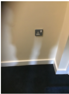
Electrical sockets provided in common parts.
