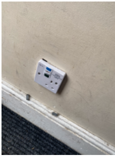
Electrical socket in the common area
