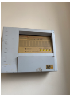
Fire alarm panel with no power supply evident.
