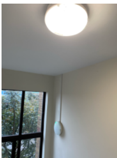
Maintained EL is provided in the staircase and lobbies.
