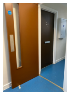
Lobby doors wedged open
