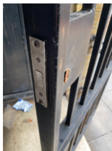
Mortice lock in security gate fitted externally across main entrance door
