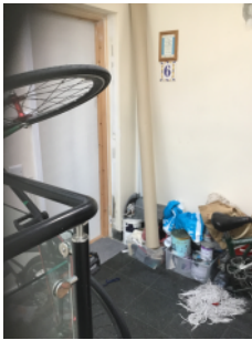
Combustibles in the staircase
