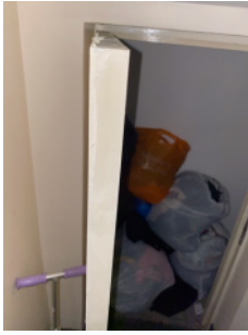
Under-stairs cupboard door should be FD30S
