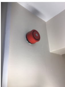
Fire alarm sounders provided in common areas.
