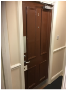
Example of FED provided in the building.
