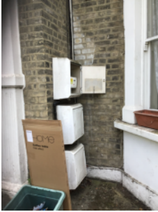
Gas meters located externally
