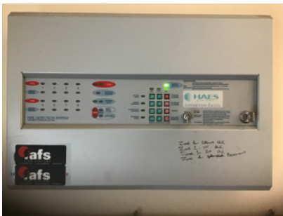
Fire alarm panel
