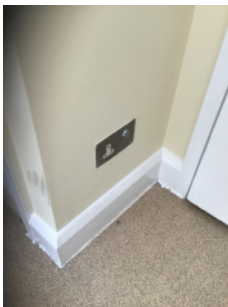
Electrical socket provided in common staircase
