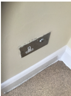
Electrical socket provided in common staircase.
