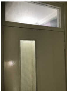
Georgian wired glazing
