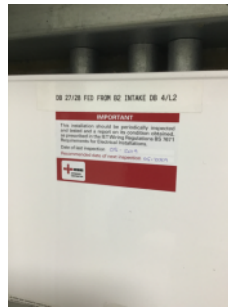
Example of test labels on electrical installations
