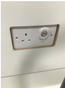
Secured cleaners electrical sockets in common areas.
