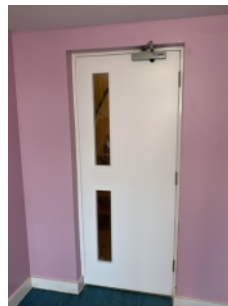
Escape route FROM ISHA offices - no exit available via this door.
