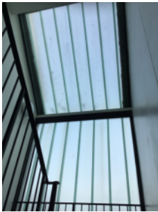
Construction in staircase - no smoke ventilation
