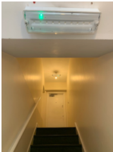
Non-Maintained Emergency Lighting units on ground and first floors.
