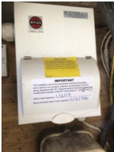
Evidence of testing of fixed electrical installations in external cupboard
