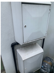
Gas meters located externally
