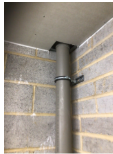
Large soil pipe penetration in the bin store without fire stopping
