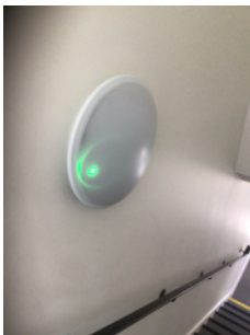
Maintained EL provided in common escape routes.
