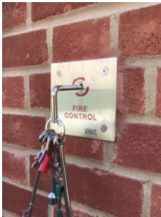
Fire service override device tested and working correctly
