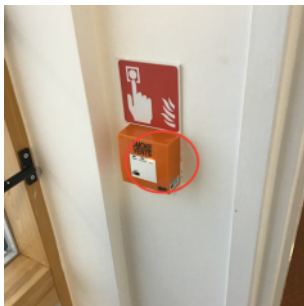
Fault light on smoke vent actuator
