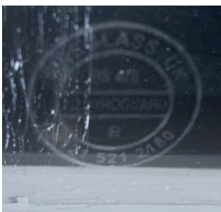
“Pyroguard” FR Glazing in corridor doors.
