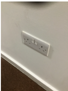
Electrical sockets in common areas
