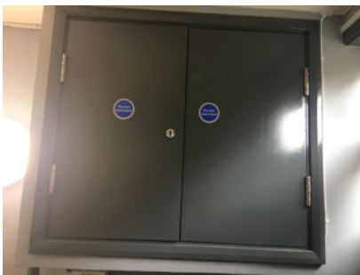
Signage provided on the electrical cupboard door.
