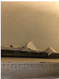
Fire stopping required around inside of electrical cupboard doorframe
