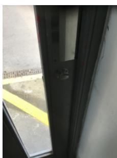
Thumb turn device provided on main entrance door.
