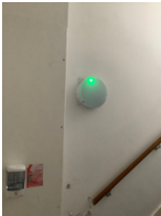
Maintained EL in the staircase
