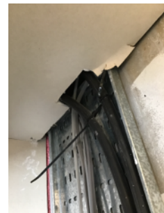
Lack of effective fire stopping inside electrical cupboards
