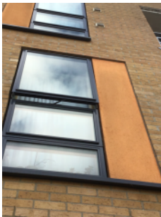
Rainscreen panels on windows
