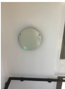
Maintained Emergency Lighting in the staircase
