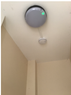
Emergency lighting in hallway
