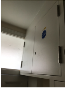
Fire resisting enclosure around electrical installation
