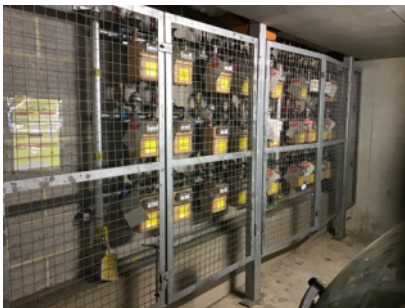
Gas meters located within the undercroft carpark
