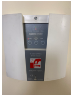
Smoke vent control – showing fault and alarm.
