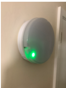
Maintained EL within corridors, and the staircase
