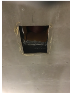
Breaches of the undercroft carpark ceiling
