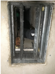
Breaches of the undercroft carpark ceiling
