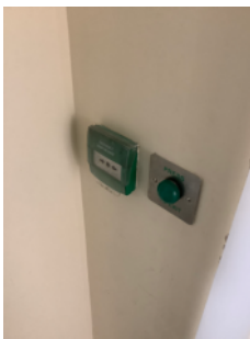
Electromagnetic door release with emergency override, staircase doors
