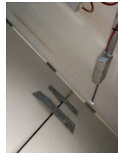
Opening mechanism at the rear of the smoke shaft door has become detached.
