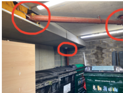
Large pipe penetrations without fire stopping within the bin store.
