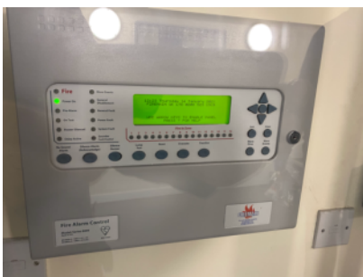
The fire alarm panel.
