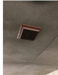
Breaches of the undercroft carpark ceiling
