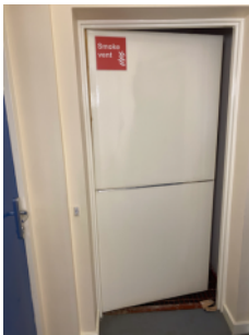
Defective smoke shaft door on the first floor.
