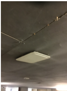
Breaches of the undercroft carpark ceiling
