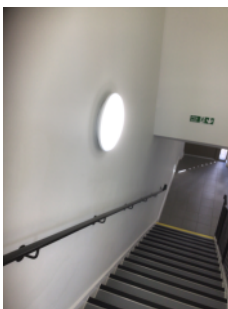
Maintained EL provided in common escape routes.
