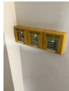
Smoke controls inside main entrance, ground floor
