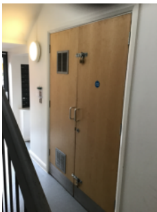
Access could not be gained through this door, ground floor entrance hallway
