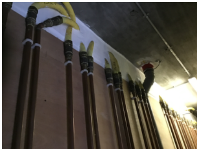
A good standard of fire stopping within the gas meter room.
