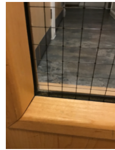
Acid etching on glazing within doors.
