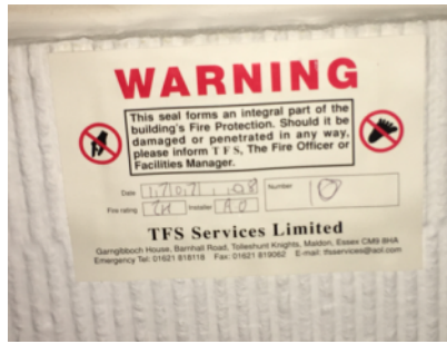
Example of fire stopping label within riser cupboards.
