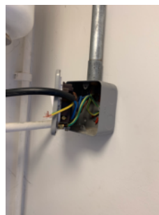
Exposed wiring by bad practice from on site contractors.
