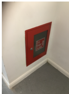
Dry rising main
