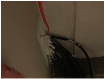
Example of fire stopping within riser cupboards
