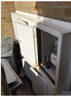
Unlocked gas meter cupboards
