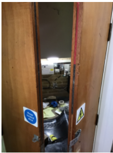
Missing strips and seal
