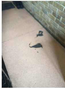
It is evident that a small fire has occurred on the 2nd floor landing.
