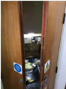
Unlocked electrical cupboard
