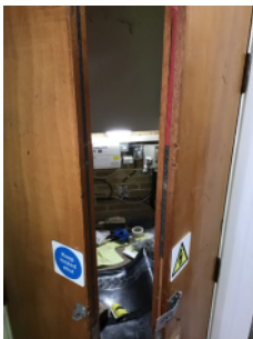
Combustibles in electrical cupboard
