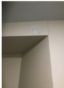
Holes in walls should be properly repaired.
