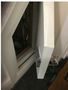
FD30S door to the electrical cupboard
