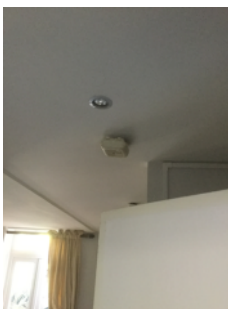
Smoke alarm in flat entrance hall.
