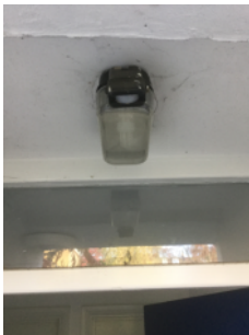
External porch light with PIR.
