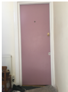
FED on first floor.
