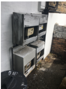
Gas meter cabinets- require repair
