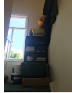
Combustibles in the common area.
