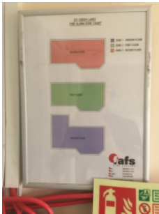
Fire alarm zone information
