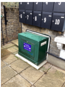
Gas meter externally
