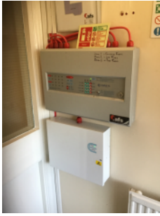
Fire alarm panel with separate battery casing (suggests Grade A)
