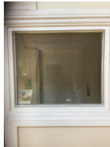
Georgian wired glazing installed in lobby partitions
