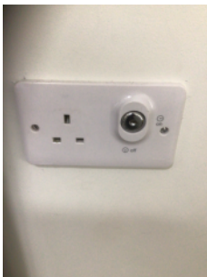
Key isolated electrical sockets are provided.
