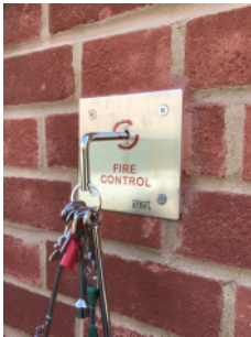
Fire service override device tested and found defective
