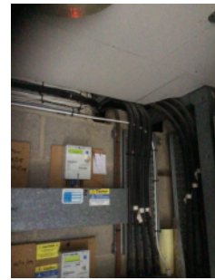
Cable penetrations within the electrical meter cupboard.
