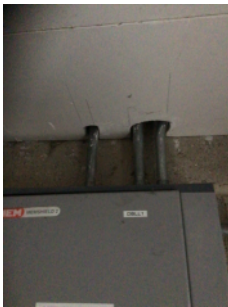
Cable penetrations within the electrical meter cupboard.
