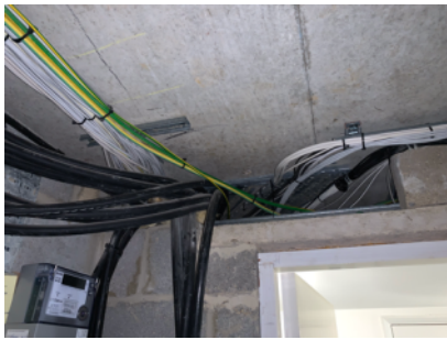
Cable penetrations in electrical intake cupboard require fire stopping
