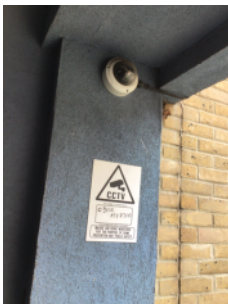
CCTV cameras are located internally and externally
