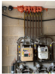
Expanding foam should not be used on penetrations of this size
