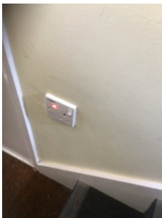
Electrical socket located in the staircase.
