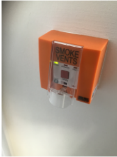
Smoke vent control showing power supply with no fault evident
