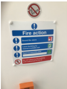
Incorrect Fire Action Notice for the stay put policy in place
