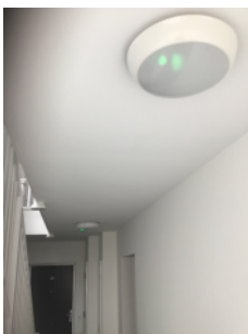
Maintained EL (local) is provided in the staircase
