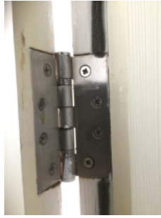
CE Marked fire rated door hinges on riser doors
