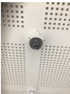
CCTV cameras are provided internally and externally
