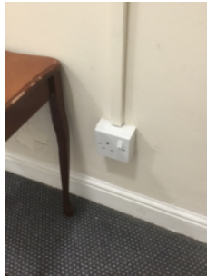
Power outlet in common area.
