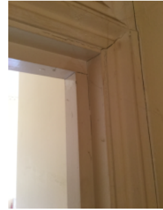
25mm door stops to internal flat doors.
