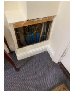
Missing hatch cover exposing wiring in entrance hallway.
