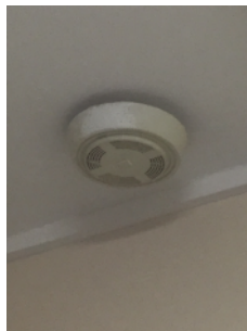
Part 6 smoke alarm in staircase.
