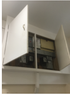
High-level electrical cupboard.
