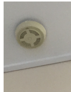
Part 6 smoke alarm in ground floor hallway.
