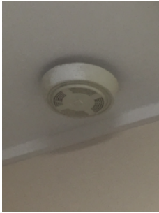
Part 6 smoke alarm on first floor landing.
