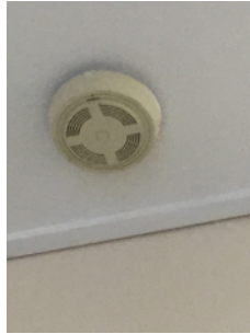
Part 6 smoke alarm on ground floor.
