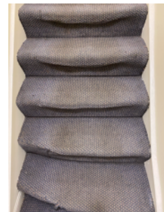
Loose carpet over stair nosings.
