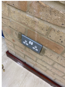
Electrical sockets provided in common areas
