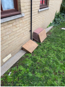
Gas meters located externally
