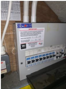
Evidence of testing of fixed electrical installations - electrical cupboard
