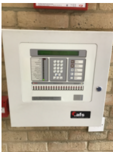
Fire alarm panel
