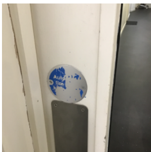
Fire door signage requires replacing
