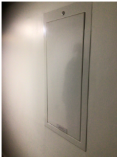
Example of Smoke shaft door in corridors
