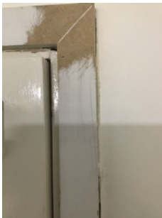
Corridor door not closing fully into frame.
