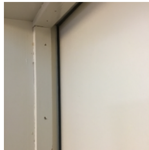
Corridor door not closing fully
