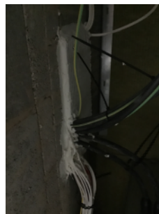
Example of fire stopping within riser cupboards.
