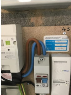
Valid test labels on gas meters
