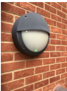
Maintained EL in external areas
