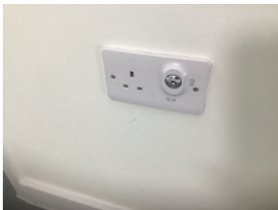
Electrical socket with isolating lock
