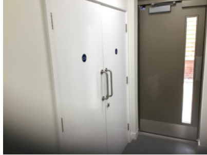
It was not possible to access these doors.
