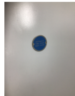
Automatic self-closing fire door signage
