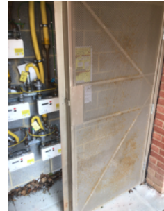
Gas meter is located behind a vented doors.
