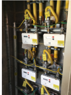
Gas installations in secured externally accessed enclosure
