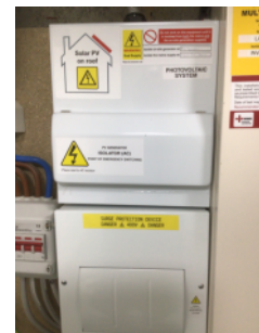
Photovoltaic generator isolator located in first floor riser cupboard
