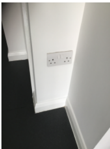
Electrical sockets provided in common areas
