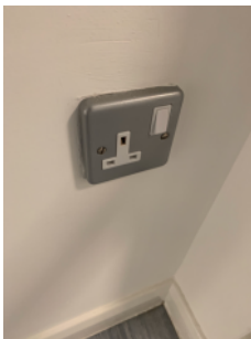
There are electrical sockets in the common areas
