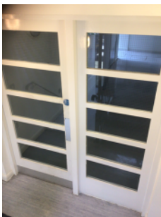
Georgian wired glazing on the staircase.
