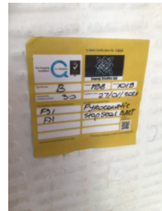
Fire stopping certifying label within riser cupboards.
