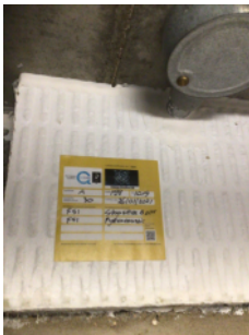
Fire stopping certificated label in ground floor electrical cupboard
