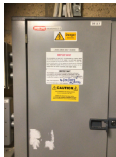
Evidence of testing of landlords distribution board
