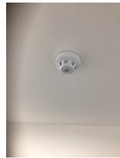
Smoke detection in corridors for the actuation of the smoke ventilation.
