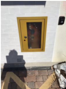
Dry riser inlet
