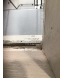
Acid etching on FR glazing installed in the staircase doors
