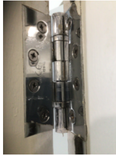
Hinges to EN1935:2002 standard fitted in staircase doors
