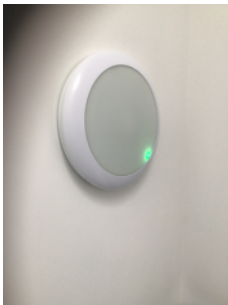
Maintained EL in the staircase
