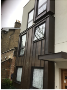
Metallic ring screen and front face of building and around window openings External wall details
