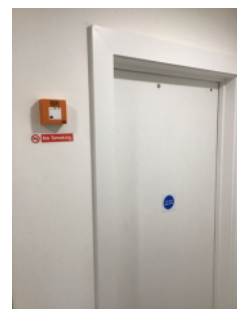
Wrong signs on smoke vent signs
