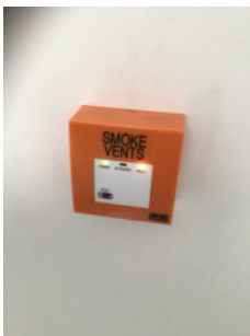
Smoke vent actuators showing in a fault condition
