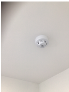
Smoke detection in staircase for the actuation of the smoke ventilation.
