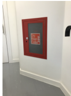
Dry riser outlet on each landing
