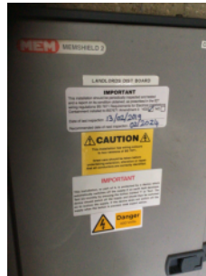
Evidence of testing of landlords distribution board.
