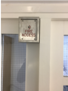
Firefighters override on lobby doors.
