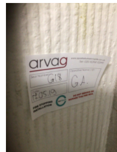
Fire stopping certifying label in riser cupboards.
