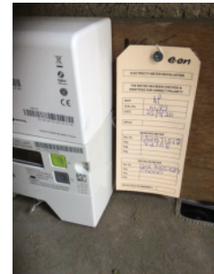
Evidence of testing of resident's electricity meters.
