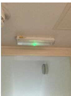
Non-maintained emergency lighting in staircase.
