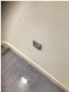
Electrical sockets are provided in common areas.
