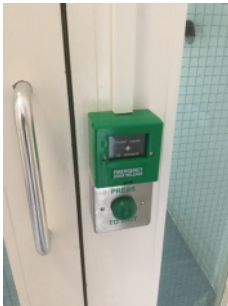
Override buttons on lobby doors.
