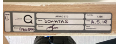
BMTRADA fire door certification on riser cupboard doors
