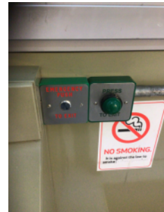
Electromagnetic door release and emergency door release, main entrance door
