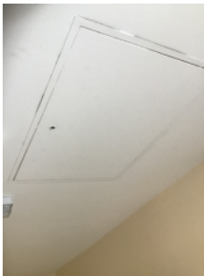
It was not possible to access the loft space within the scope of this FRA
