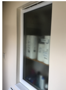
Internal glazing in the lobbies does not appear to be FR.
