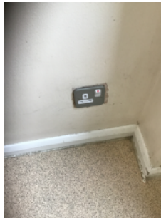
Electrical sockets in common areas
