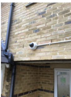
CCTV is provided externally
