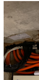
Fire stopping within the electrical cupboard
