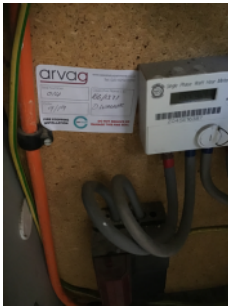
Electrical installations tested in September 2019.
