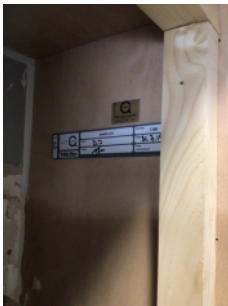
FR Certification label within electrical cupboard
